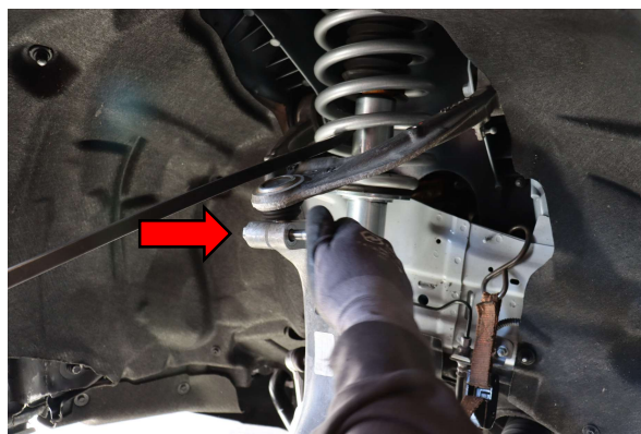
Step 21. Using a pry bar, lower the upper control arm ball joint into the top of the spindle. While pulling down on control arm, install 16mm nut and bolt in top of spindle. Tighten to factory specification. Remove the strap used to support the spindle during shock replacement.
