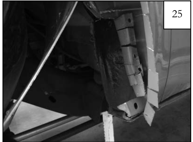
Inner flange flush against wheel well wall.
