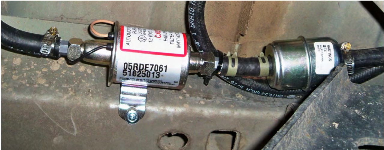
(Fig. 14) Fuel pump and inline filter installed.
